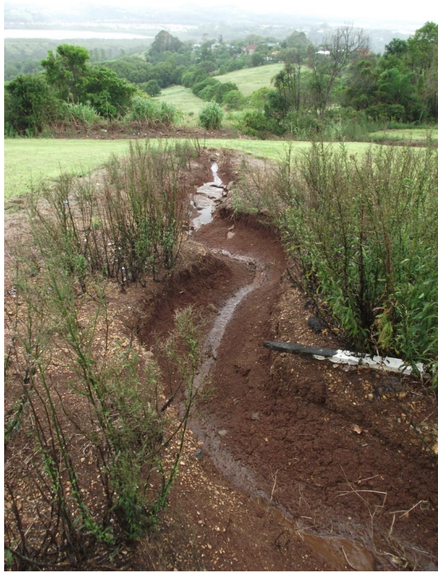
Figure 6 – Existing Scoured Drainage Line below Pipe under Terranora Road
